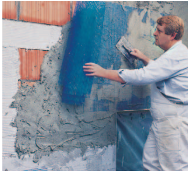
Fig. 22: Applying floating and fiberglass reinforcement mesh on top of insulated concrete units.
