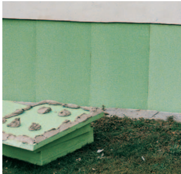
Fig. 31: Reconstruction of an old building: Styrodur 2800 C boards are applied (dot-and-bead application).
