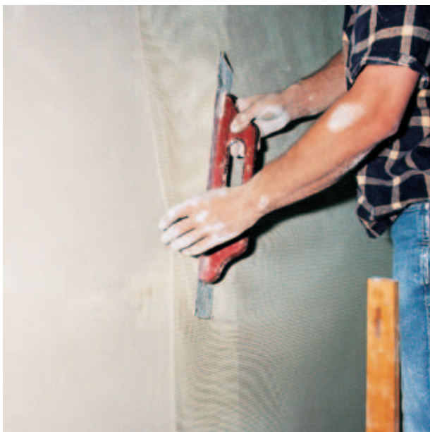
Fig. 33: Applying the fiberglass reinforcement mesh on the whole surface. The layers should overlap approx. 100 mm.
