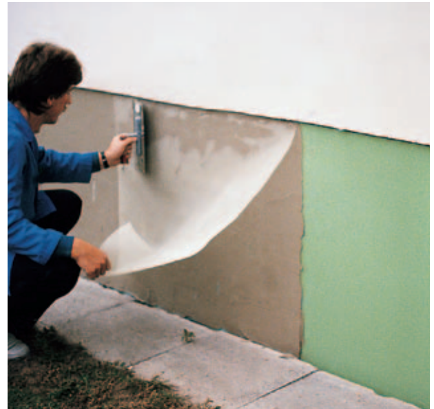
Fig. 29: Application of the fiberglass grid on the plaster foundation of the base course.
