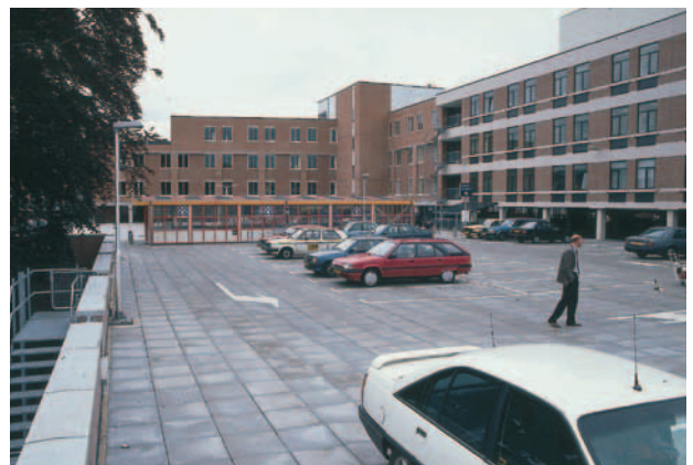
Fig. 45: Parking roof with concrete slabs laid on an inverted roof with Styrodur C.
