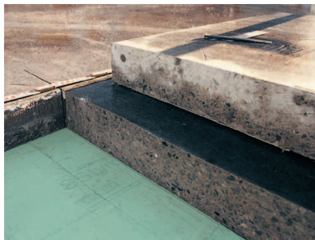
Fig. 52: In-situ concrete driving surface slab, sliced for the scientific examination of its long-term behavior.
