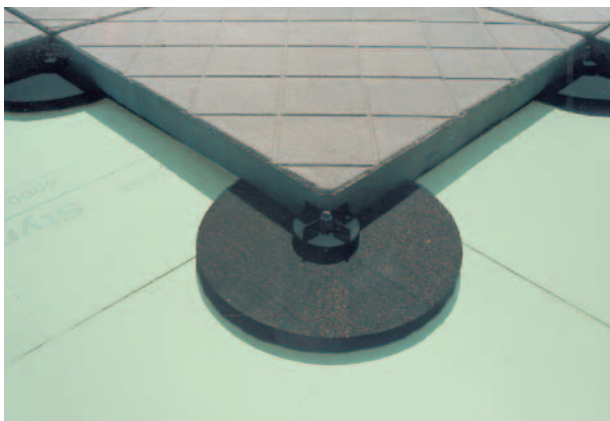
Fig. 44: Concrete slabs laid on Styrodur® C using a pavement slab support system.
