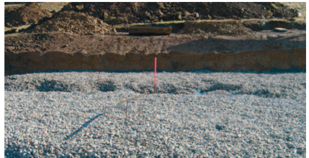
A gravel bed as a blinding layer and leveling plane makes for a flat base. This base course is prepared according to the requirements of the building ground and the instructions of the structural engineer.
