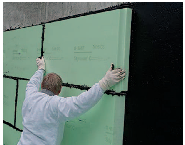
Fig. 17: Attaching the Styrodur® C boards and sealing the joints against pressing water.
