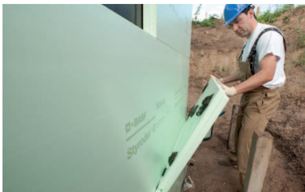
Fig. 5: Point bonding the second layer of Styrodur C boards with overlap and offset joints.
