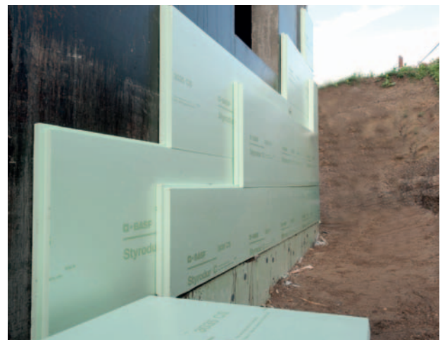
Fig. 3: Securing a two-layer perimeter insulation of Styrodur® C boards until the backfilling of the excavation pit.
